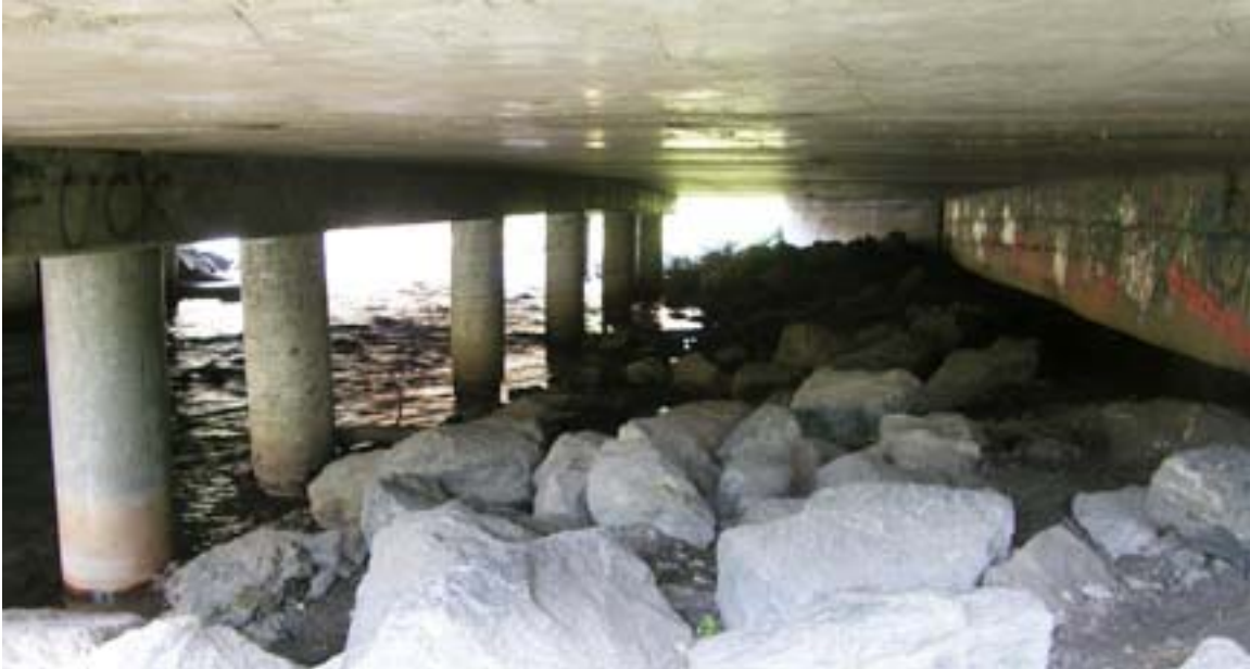
View from East along north embankment where proposed underpass would be built.
