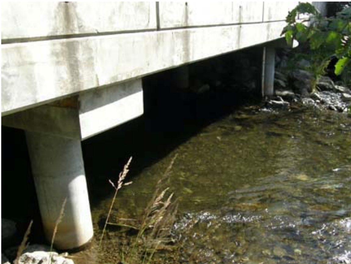
Campbell Cr. flowing from the west portal of Lake Otis bridge between support columns.
